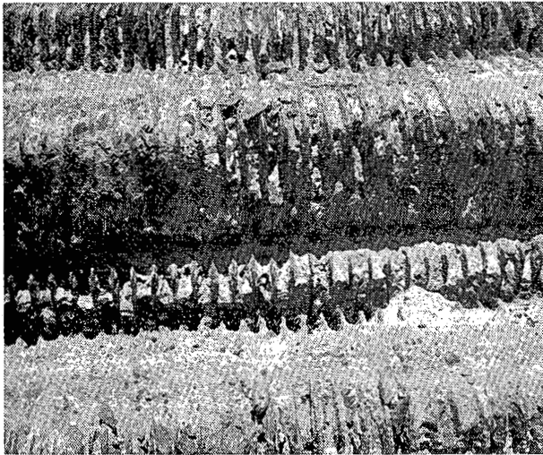
H. Economiser tubes choked with deposit. All tubes had to be removed from economiser and each one physically cleaned to bare metal. Boilers sootblown daily, economiser waterwashed every second day. Before flyash arresters fitted.
