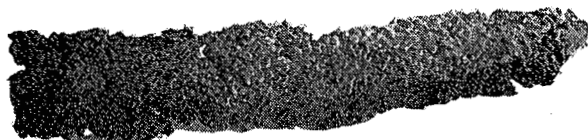
F. Deposit taken from side water wall tube showing dense but perforated deposit which has broken free from tube after being treated. Sample about 3 ft. long.
