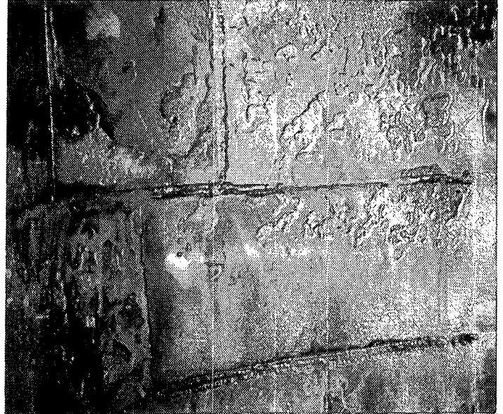
FIGURE 5 Batch pan steam chest inlet internal before epoxy coating.
