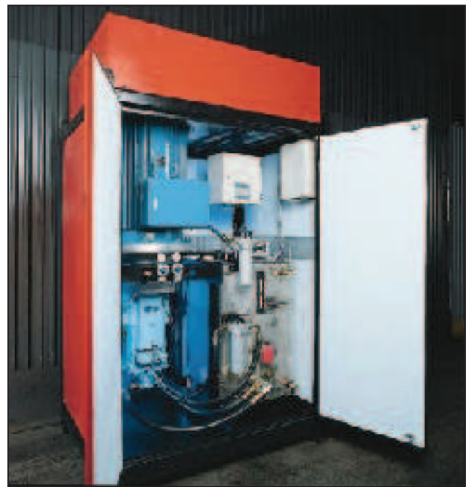
Figure 1. Photograph of drive pump and control system.
