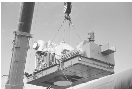
The 550-ton mobile, hydraulic boom crane (the largest in Africa) lifts the turbine / gearbox unit off the truck
