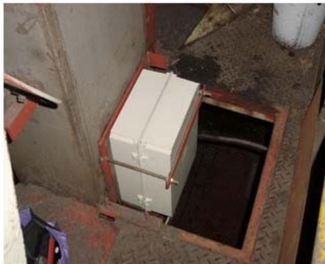
Figure 6. NIR readhead mounted in a fibreglass box bolted to the hinged window attached to the NIR chute. The window can easily be opened to clean the window or to clear bridged cane.
