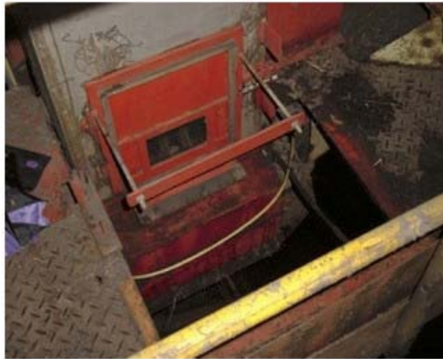
Figure 5. ‘Trapdoor’ in bottom of NIR chute with glass scanning window and mounting sill and bracket for scanhead box.
